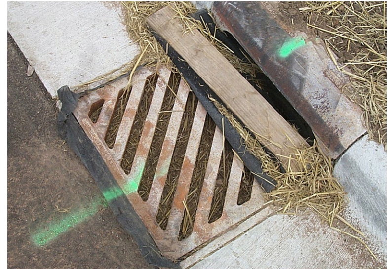
Failure to properly maintain inlet protection at construction sites increases sediment delivery to a stream
