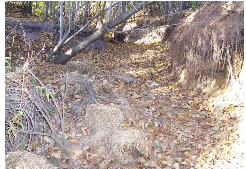
Severe erosion on a tributary to Baird Creek
